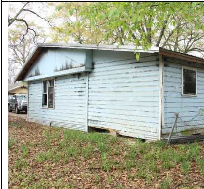
Figure 6 – Exterior rear view (Side C) of the residence after the fire.
