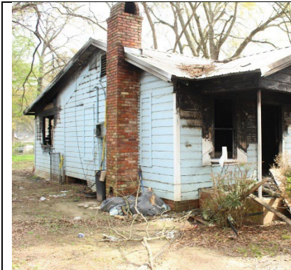
Figure 3 – Frontal (A & B sides) view of residence after the fire.
