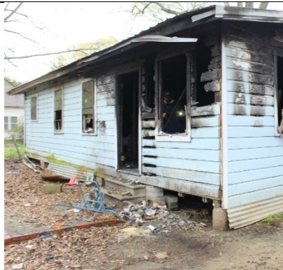
Figure 4 – Exterior side and rear view (B & C) of residence after the fire.
