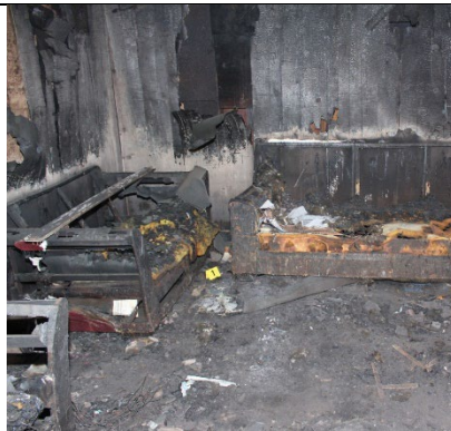
Figure 7 – Interior view of the living room where the fire was first observed after the fire
