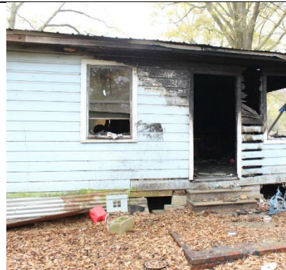
Figure 5 – Exterior rear view (Side C) of the residence after the fire where the mother exited from.
