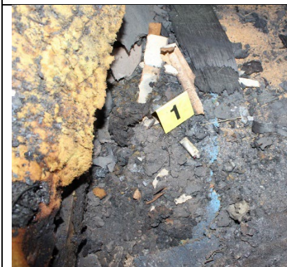
Figure 9 – The arm of the sofa where the fire was first observed. A portable lighter was observed.
